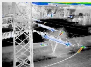
High voltage inspection
