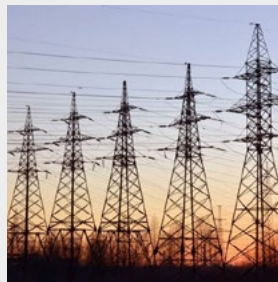
High voltage power lines
