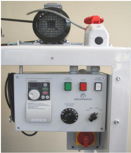
Inverter Drive Control
