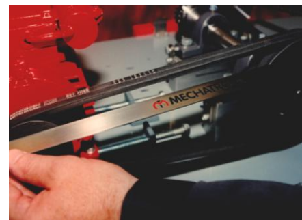
Alignment of pulleys & belts
